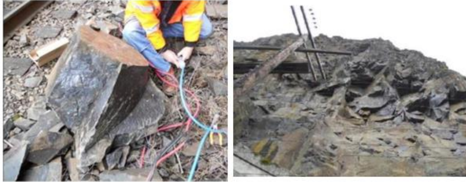
Figure 4-6 Example of 200kg rock fall - steep cliff
